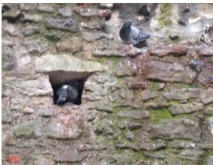
Figure 20 - Pigeons nesting in putlock holes, west elevation
